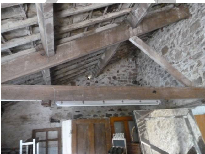
Target Note 7: Barn adjacent to house with multiple potential bat roost features, internal roof with no lining.
