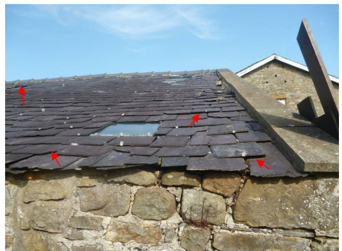
Target Note 1: Outbuilding with multiple potential bat roost features.
