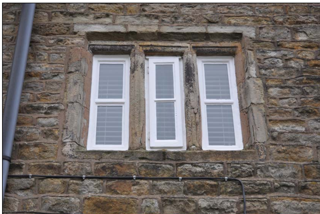
Rear window with failed mullion proposed for repair. Note poor quality cement pointing and patching
