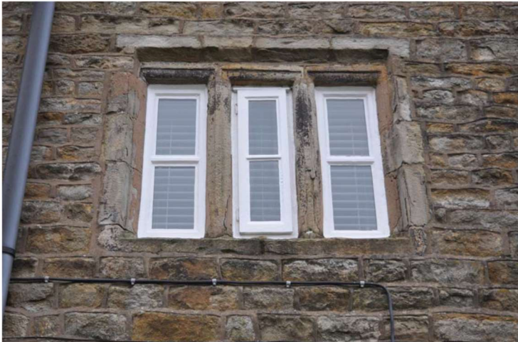
Figure 1 - Rear window with failed mullion
