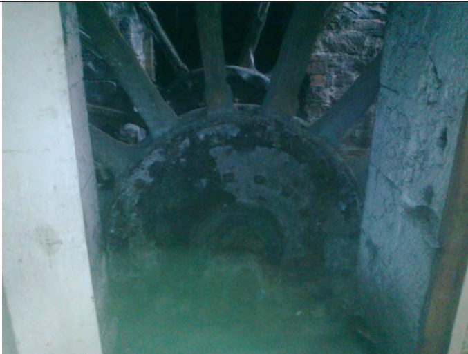
Photograph 4: Water wheel present inside the mill building.
