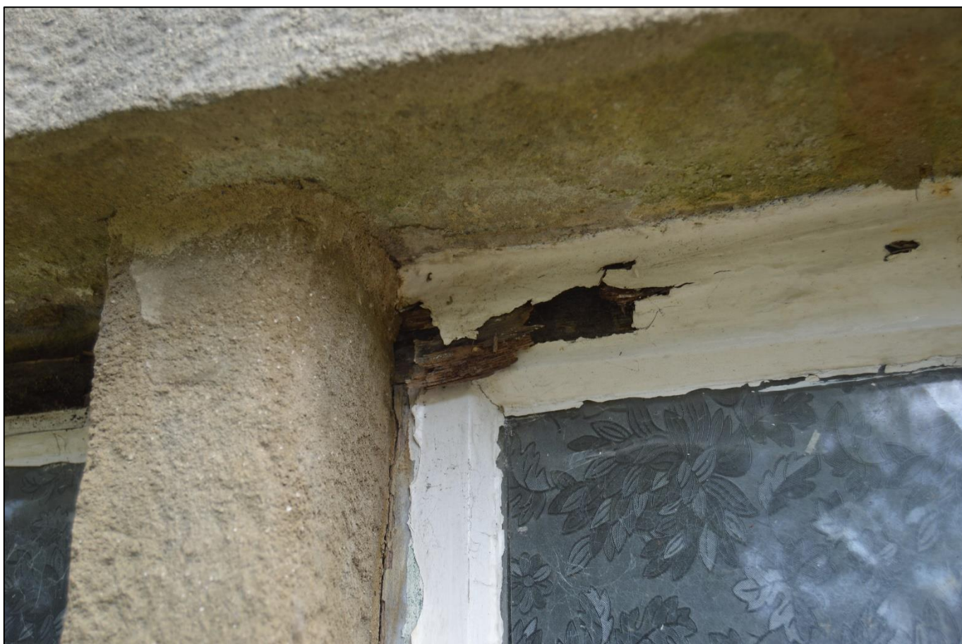
PL07: View of decay to the ground floor window to the front elevation of No. 24 Brookside.
