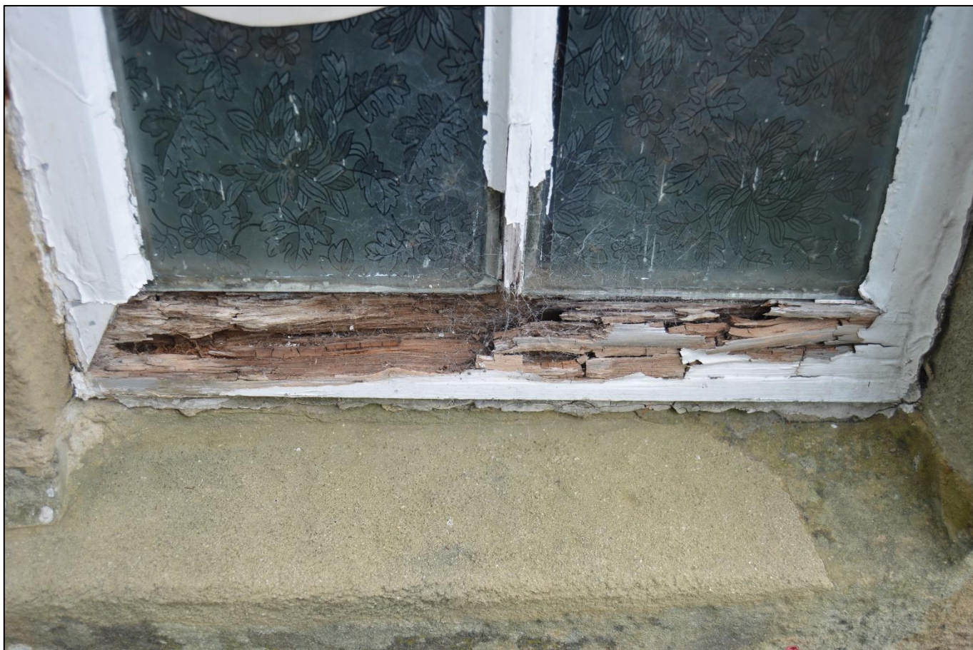
PL06: View of decay to the ground floor window to the front elevation of No. 24 Brookside.
