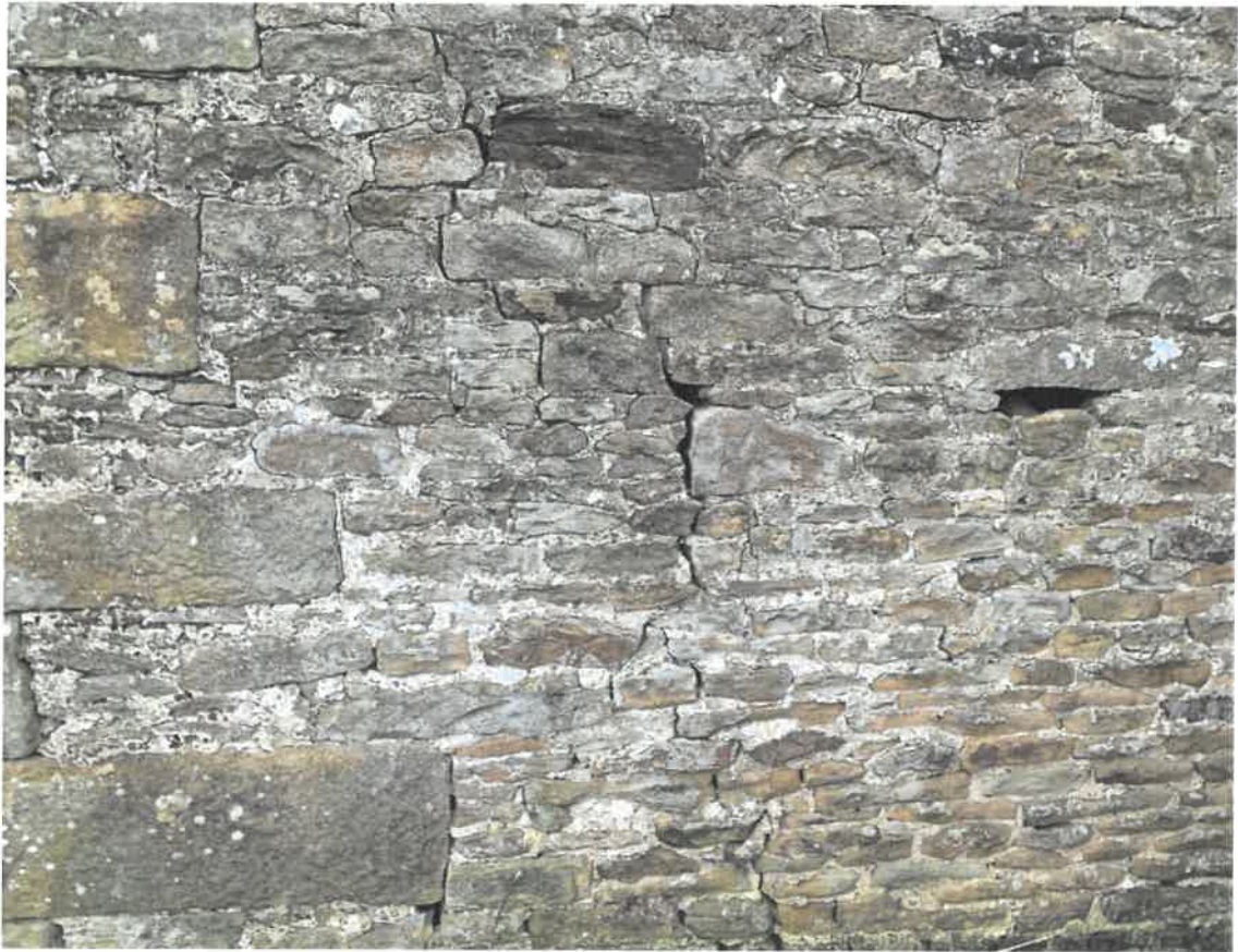
Photo 19 – east gable – Movement
