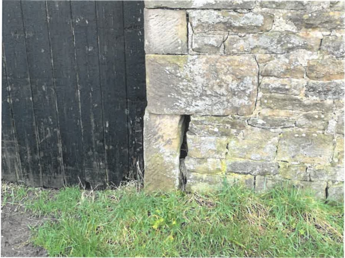
Photo 5 – North Elevation – Damage at corner of Door
