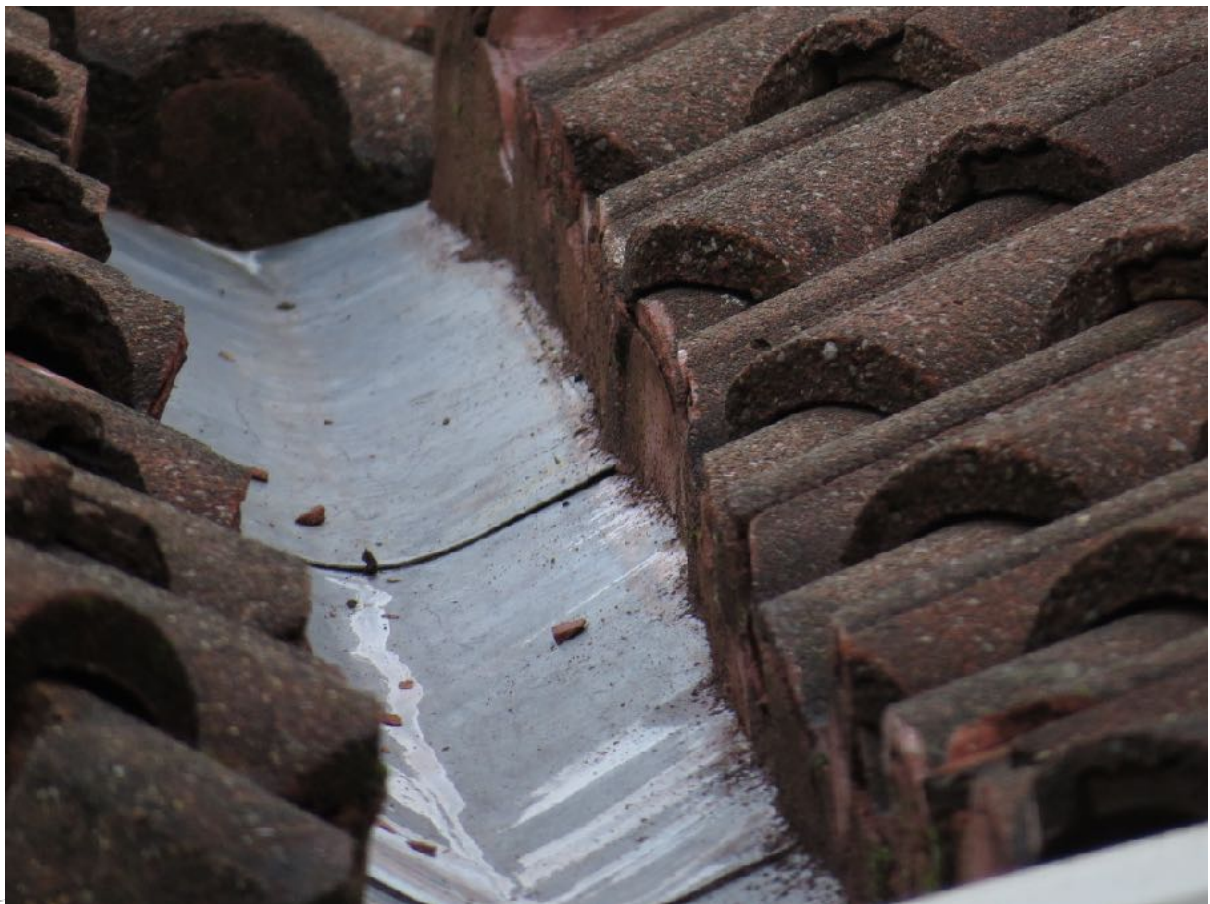
8 – End tiles in the roof valleys are filled with cement, with no suitable gaps.
