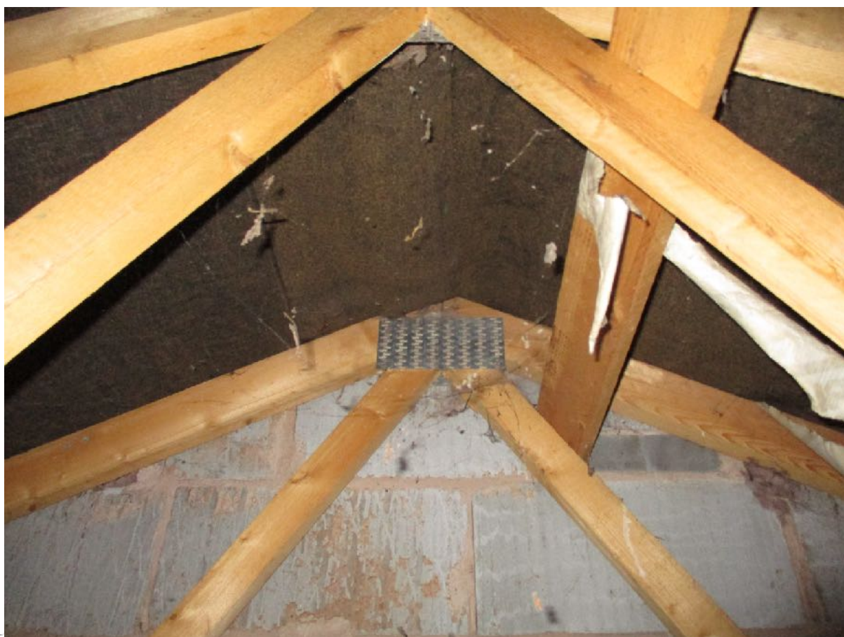
12 – Joints in timbers are filled with dusty cobwebs.
