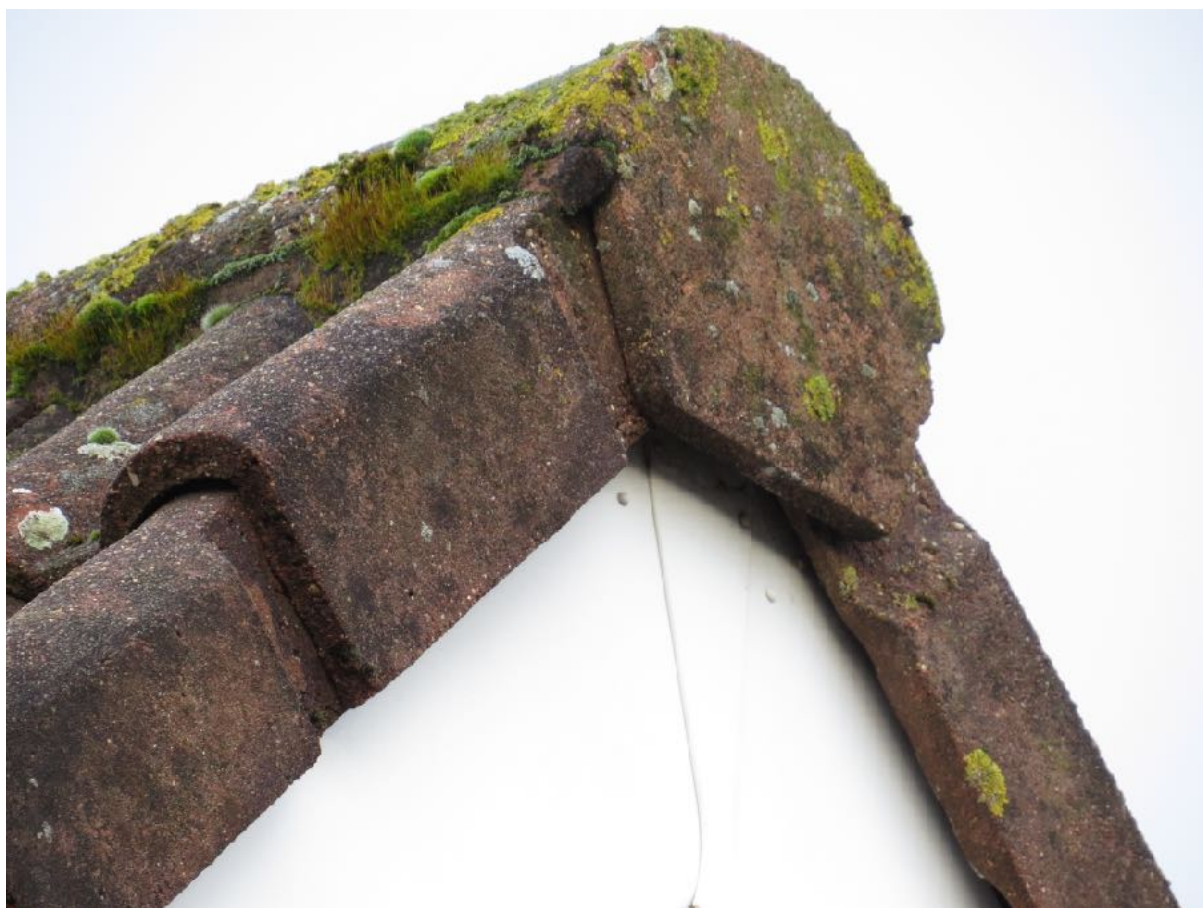
5 –End tiles at the gable end verges are sealed with no suitable gaps.
