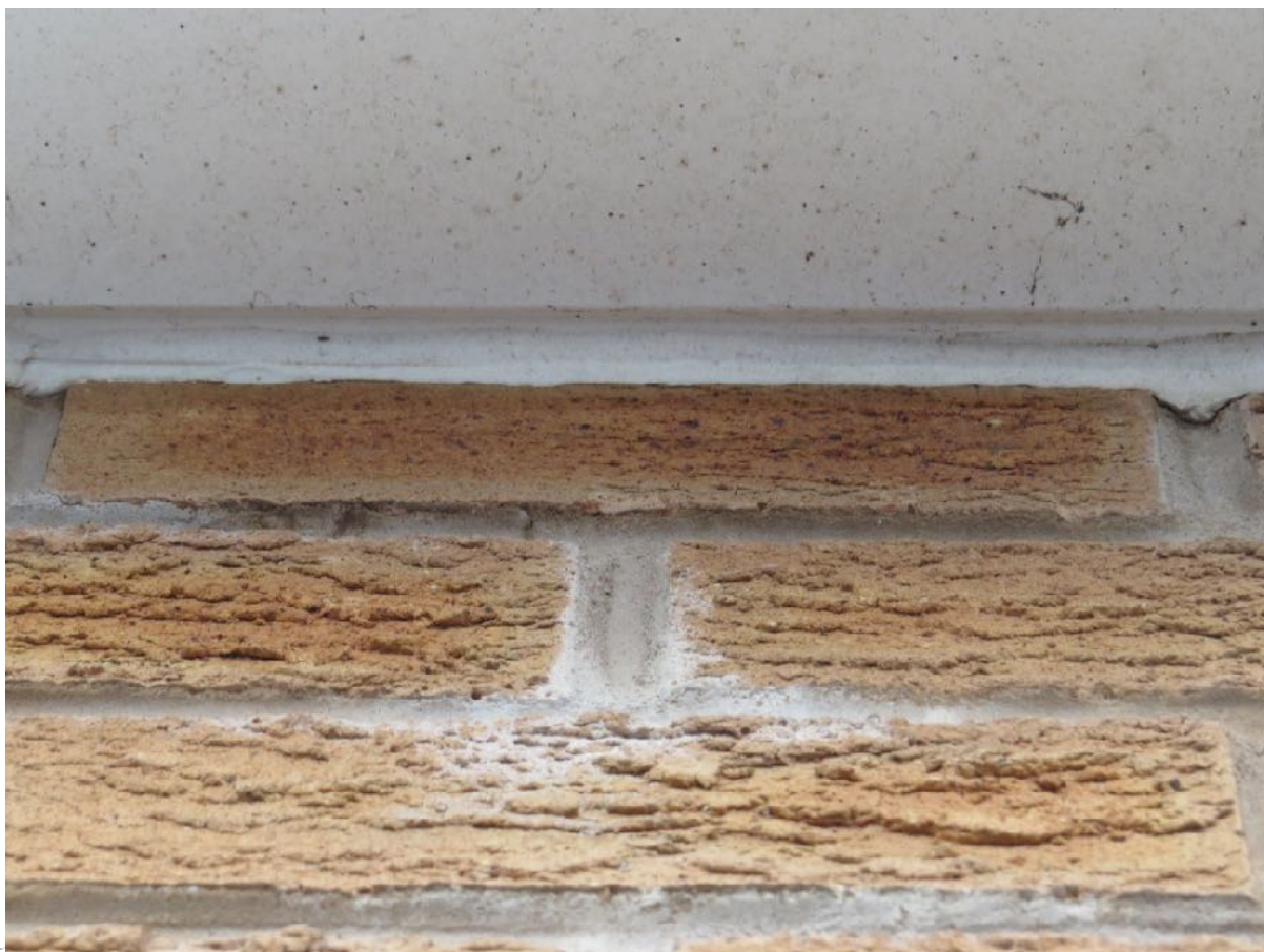
4 – Gaps between UPVC boxed soffits and brickwork are filled with sealant.
