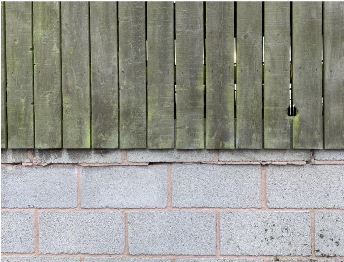
Photo 7 – North Elevation Blockwork showing minor damage
