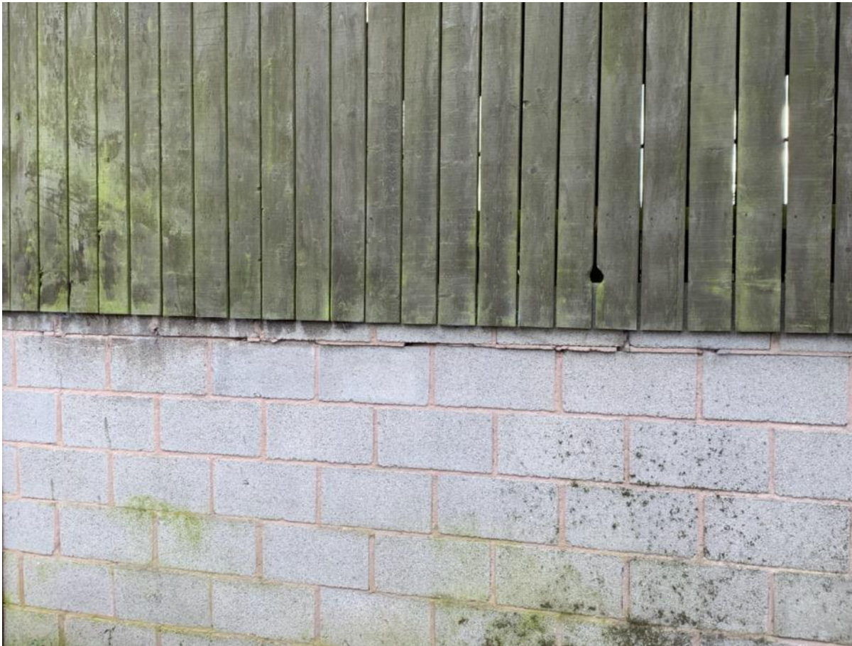
Photo 6 – North Elevation Blockwork showing minor damage
