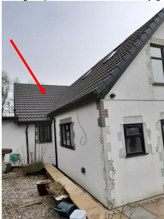
Plate 3: A photograph showing the part of the roof where the skylights will be added.
