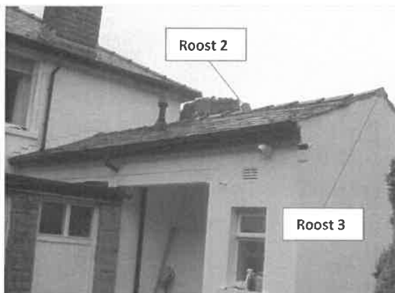
Photo 10: Single storey annex attached to the eastern corner of the house and location of Roosts 2 and 3
