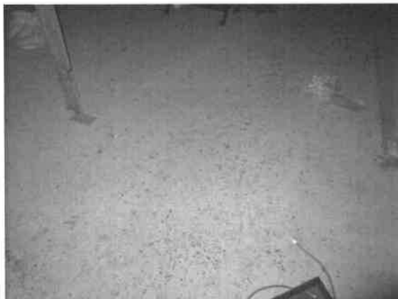
Photo 17: Scattered bat droppings over roof void of the house
