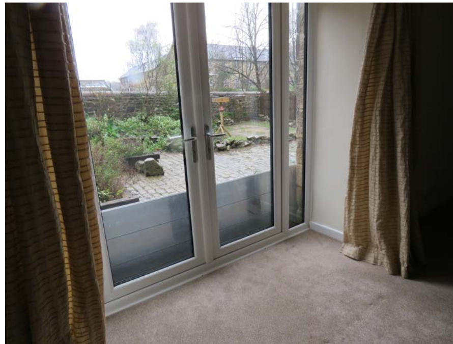
Existing UPVC doors with flood protection device installed.
