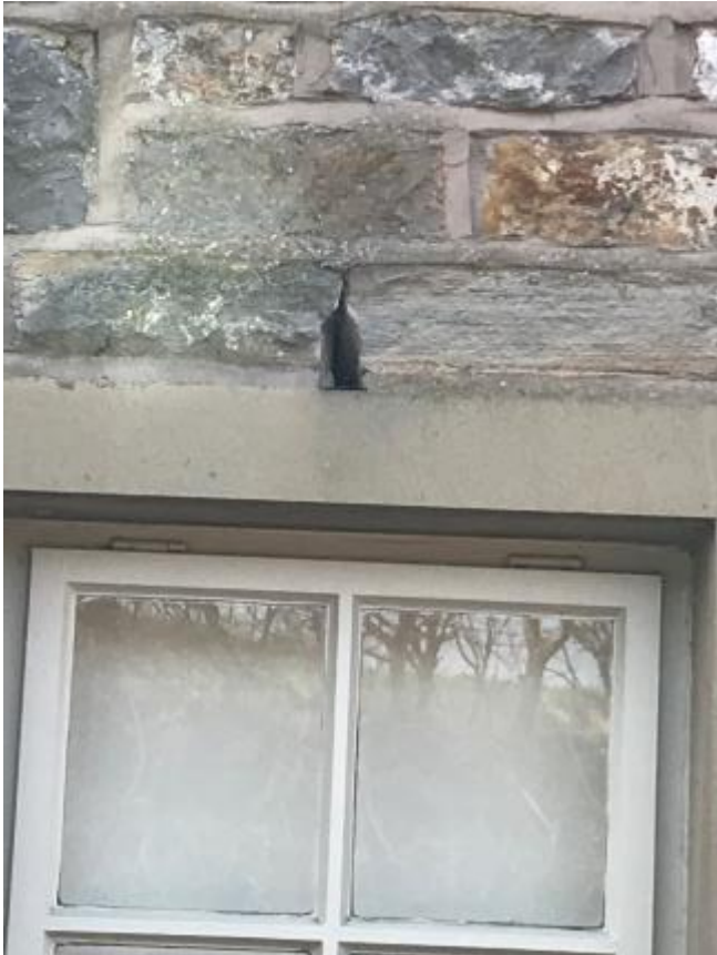
Plate 7 – Gap in the stonework above the window
