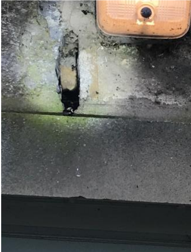
Plate 8 – Gap in the stonework
