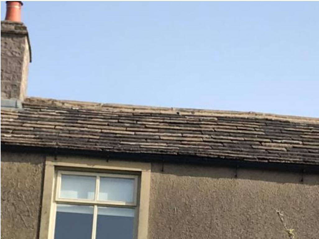
Plate 6 – Gap beneath ridge tiles on the southern elevation
