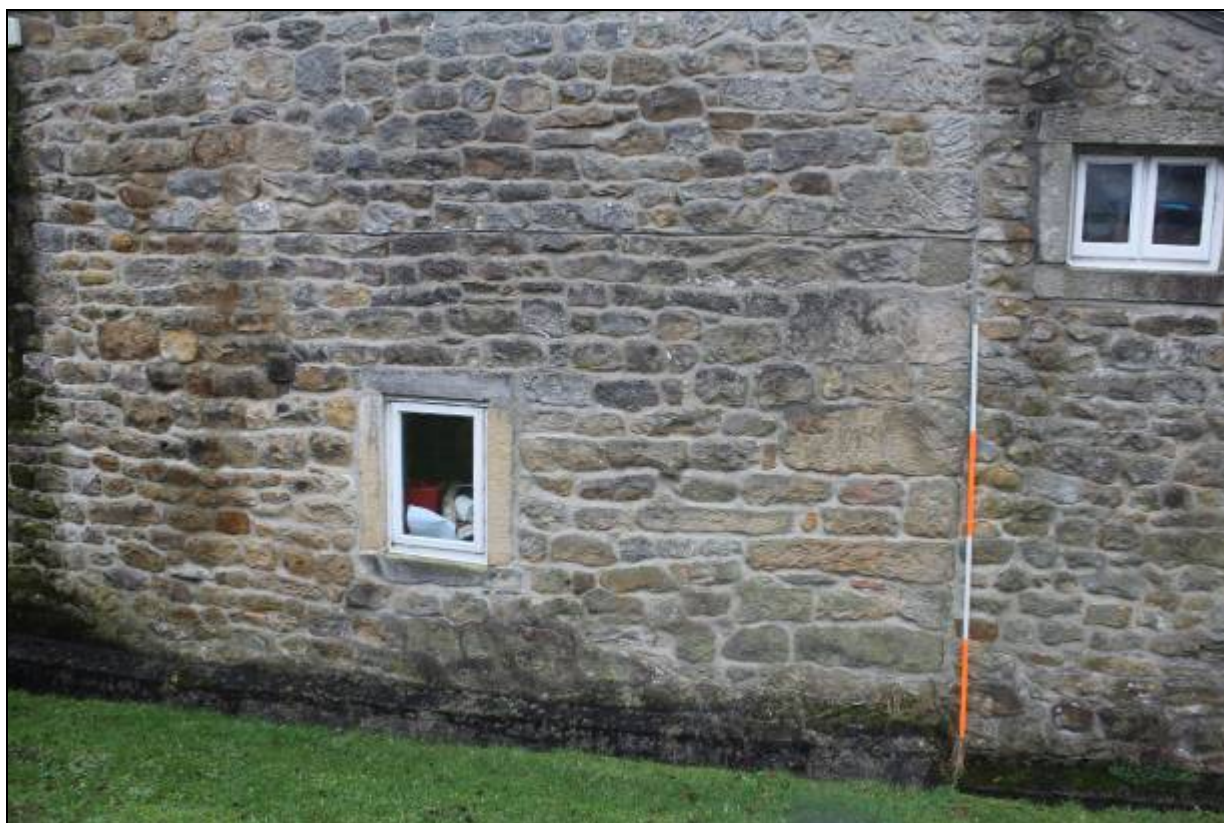
14. Straight joint on rear wall between main range and former cartshed
