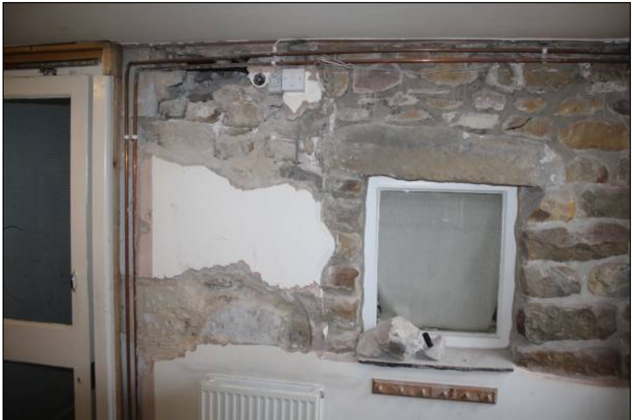
35. Former window in crosswall between first bay and cartshed (viewed from latter)
