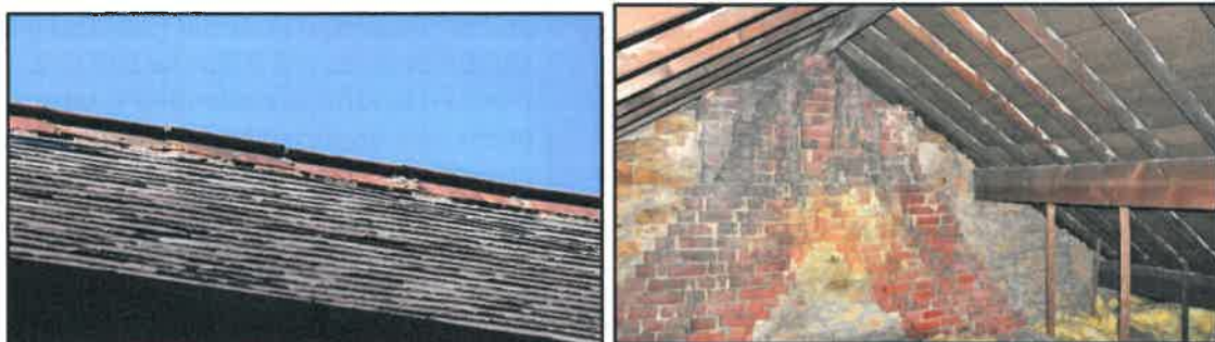
View showing roof covering with occasional gaps present between slates and ridge(lhs) and internal roof void (rhs)
