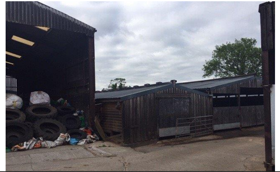
EXISTING NORTH-WEST ELEVATION THIS ELEVATION WOULD BE TOTALLY SCREENED BY EXISTING BUILDING
