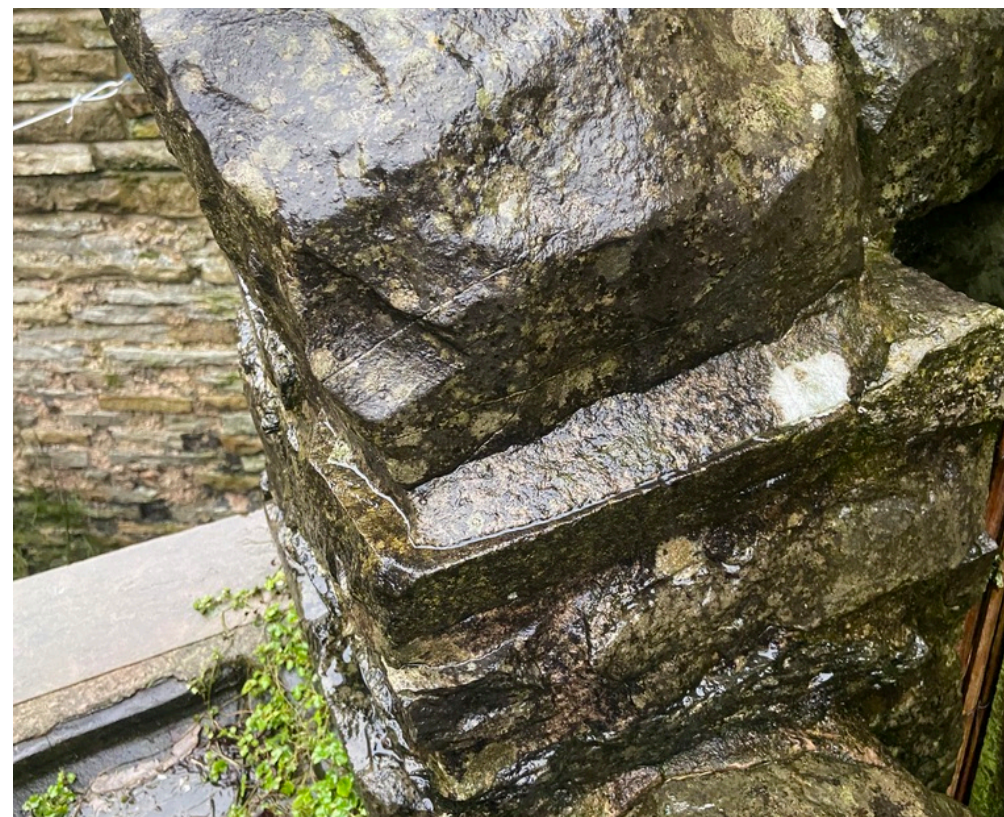
View of part of the historic Wall to the garden. This wall currently sits behind the modern outbuilding.
