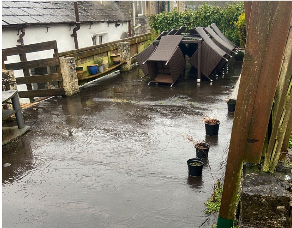
View of existing roof terrace. Note that the wooden bridge between the outbuildings and the house has since been removed.
