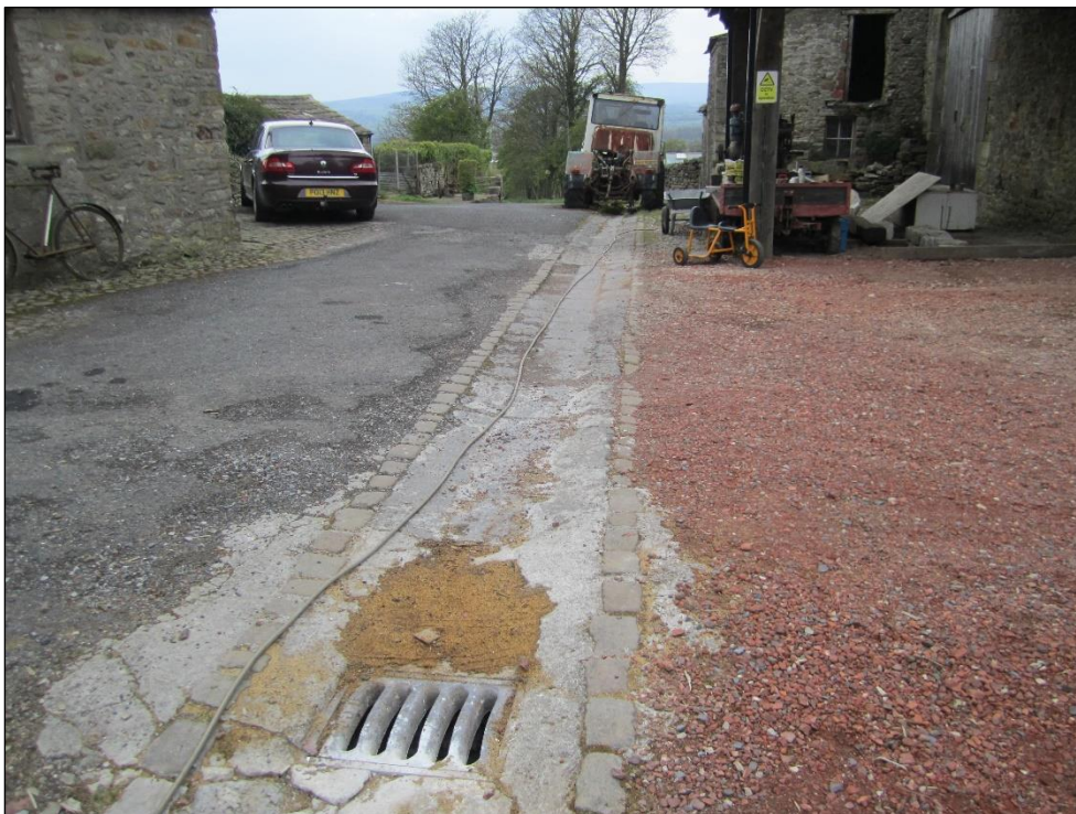
6 The gully which runs through the yard covers below surface a flat-bottomed water channel visible beneath the grid.
