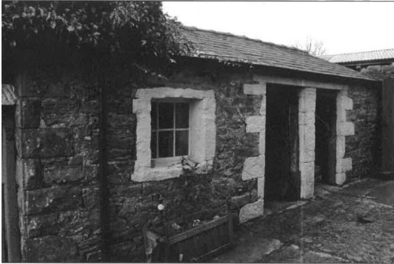
FIGURE 10: VIEW OF EXISTING OPENINGS IN OUTBUILDING 1, SHOWING OVERGROWN IVY
