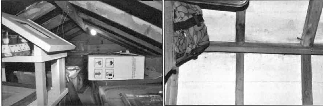
View of roof void showing shallow, cluttered space (lhs) and modern roof membrane (rhs)
