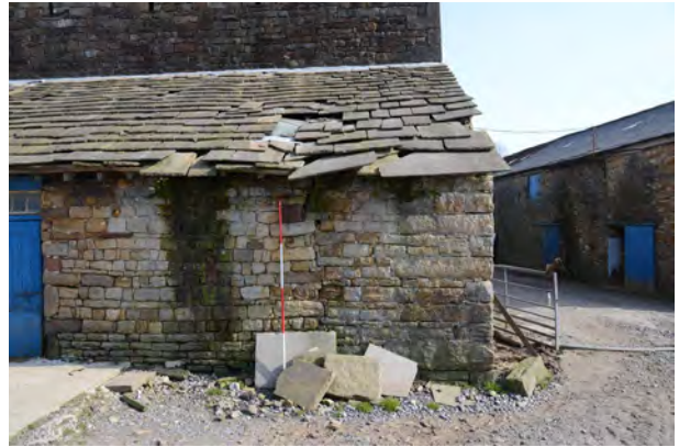
Plate 16 Vertical break in the fabric of the southwest outshut
