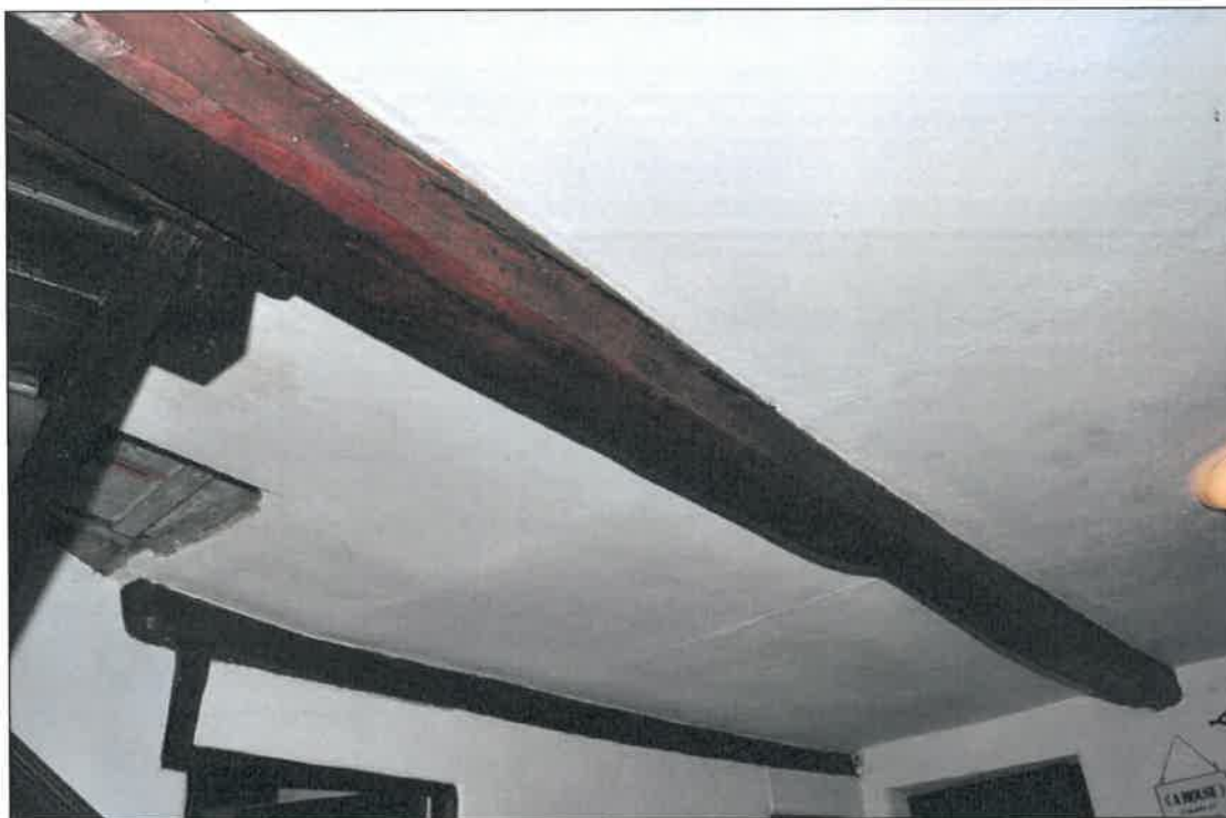
Photo 7: Beam 2, middle of lounge/living room
