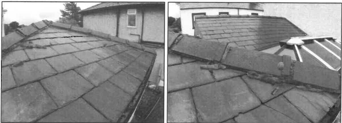
Close up view of roof coverings on single storey extension (lhs and rhs). No suitable gaps for use by bats or birds were present.
