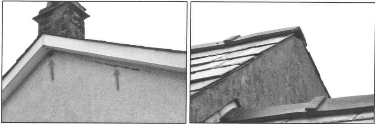
West gable of two storey section (lhs) showing tight fitting soffits with house martin nesting signs below (shown by red arrows) and west gable of single storey section (rhs) showing gap at apex with potential for use by nesting birds.
