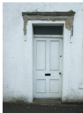
Picture 7 - Original front door with hood missing
