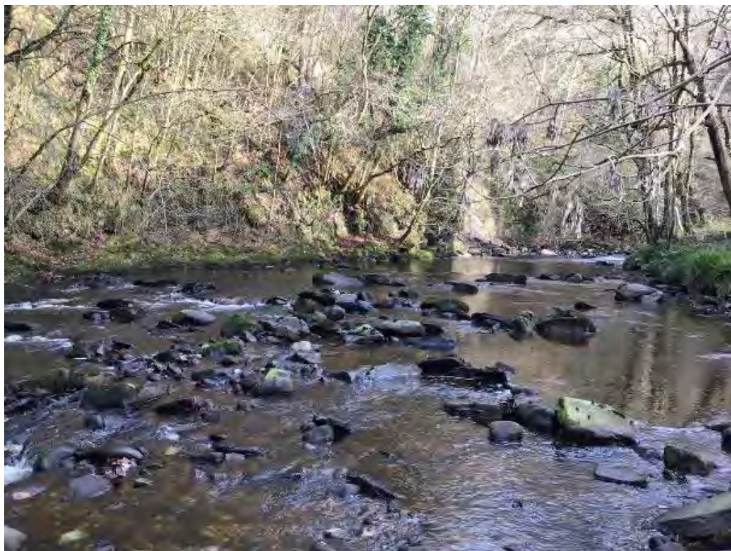
Illustration 10: Upstream view of the channel showing bank erosion on right bank
