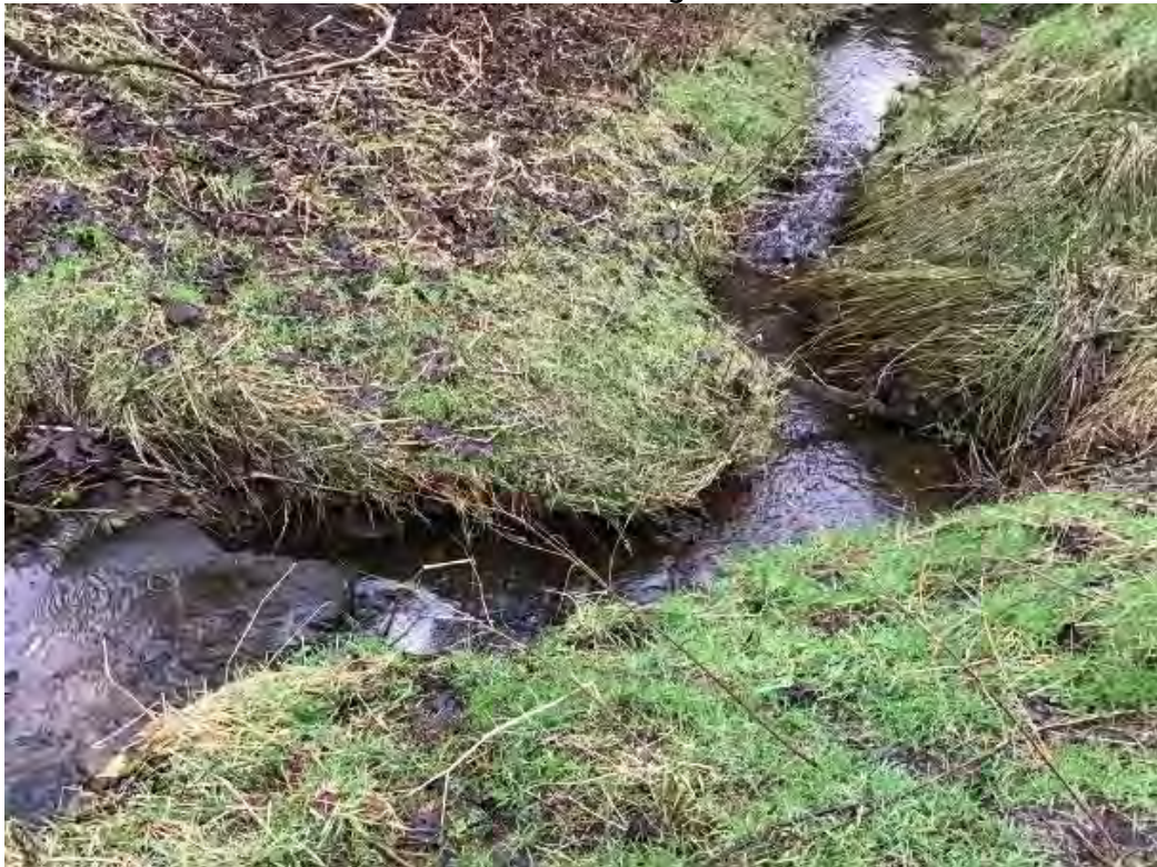
Illustration 9: Undercutting on left bank
