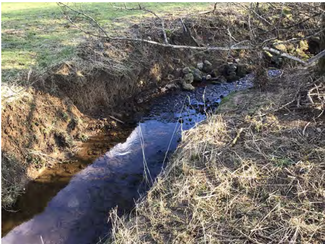
Illustration 5: Downstream view of riffle and erosion on left bank
