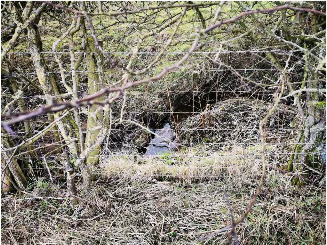
Illustration 3: View from left bank. Undercutting on right bank
