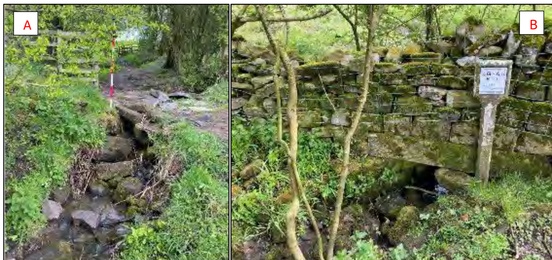
Figure 4-8: Site photographs of A: footbridge at UNN01_1781 (facing upstream), and B: boundary wall crossing at UNN01_1824 (facing downstream).
