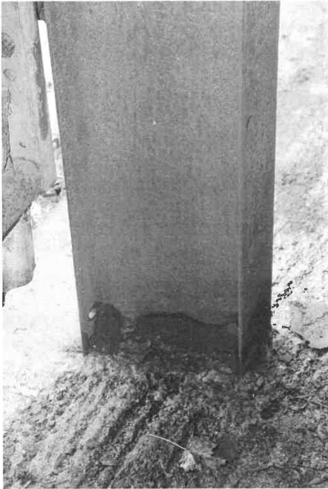
Plate 13 Showing the typical condition of a Steelwork Column at Floor Level
