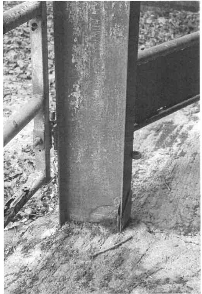
Plate 14 Showing the typical condition of a Steelwork Column at Floor Level
