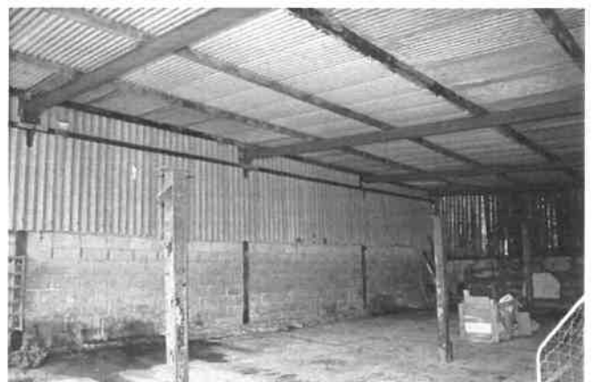
Plate 20 Showing the internal Pen area adjacent to the rear of the Barn
