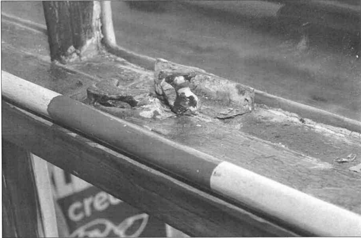
Photo 11: W1 south-west, detail of fastener
