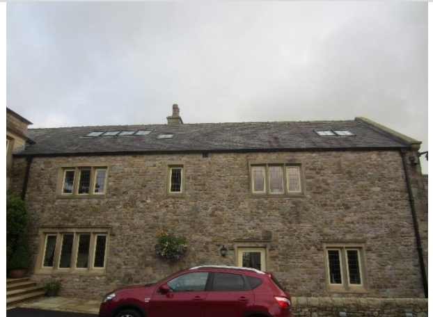
Photo 10: Northern / opposite side of property to Extension 1 showing roof pitch with skylights
