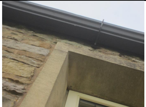
Photo 8: Gap beneath the eaves at Extension 1
