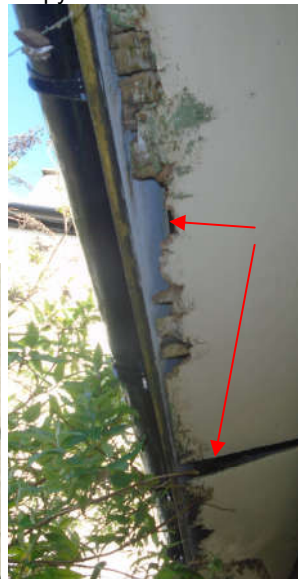
Canopy roof with rotten board
