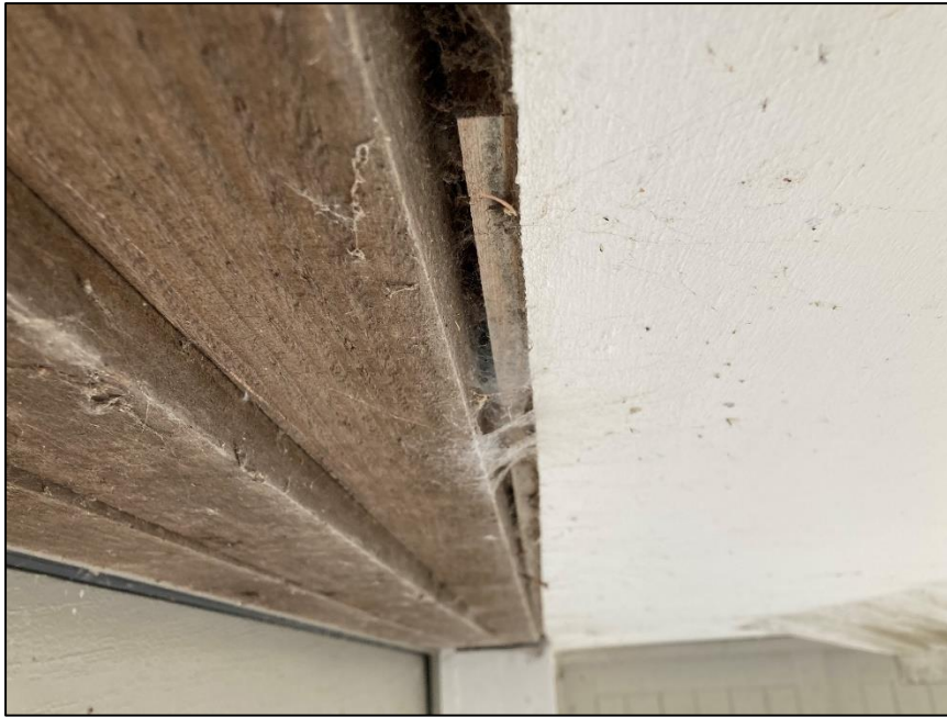
Photograph 4 showing the cobwebbed gap
