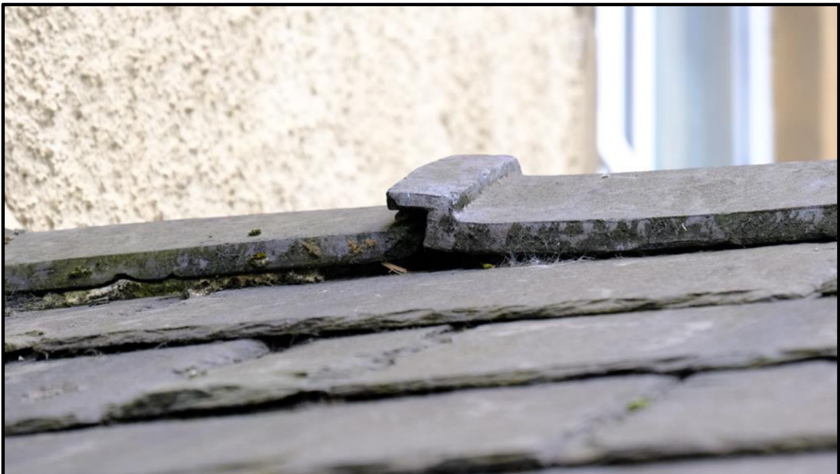
Close up view of slate roof showing example gap at the ridge
