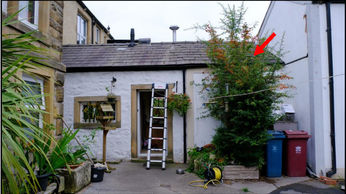
View of single storey extension (utility room) showing slate roof coverings with occasional gaps present between slates and ridge. Cotoneaster plant growing in brick planter (red arrow)
