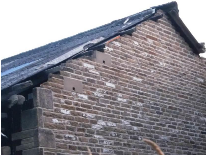
Example of Forticrete boxes in situ
