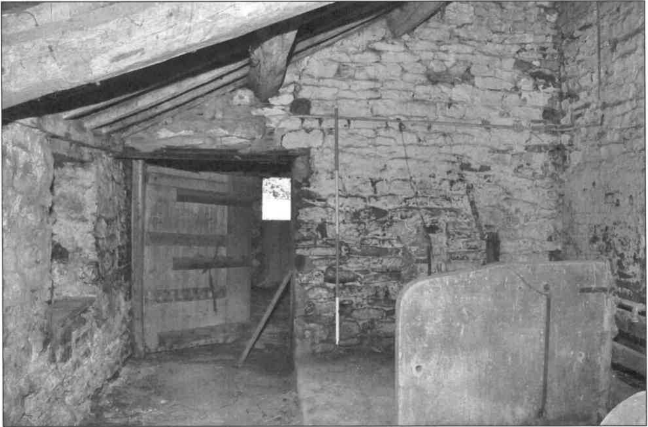
Photo 30: Outshut on north side of barn: interior of central unit, looking east
