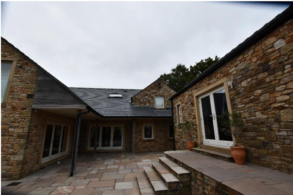
Image 2 Slight gap noted where the roof overhang meets the wall
