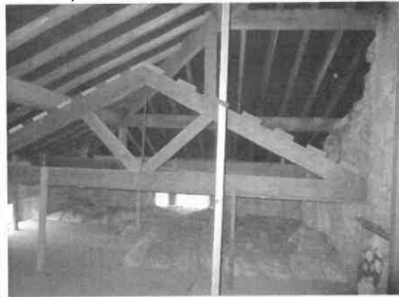
Photo 6: Roof void at Flat 8. Ceiling to be raised to the trusses as shown.
