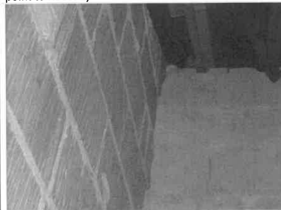
Photo 16: Accumulations of droppings on and beneath the concrete block partition wall at the top of the stair well; once inside the roof void bats have access to the hollow section of the blocks.
