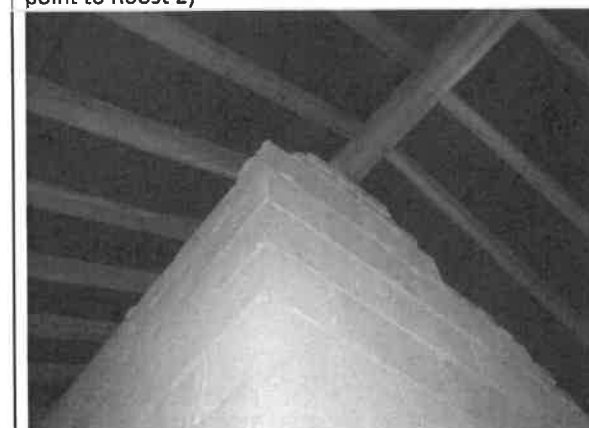
Photo 15: Concrete block partition wall at the top of the stair well; once inside the roof void bats have access to the hollow section of the blocks.
