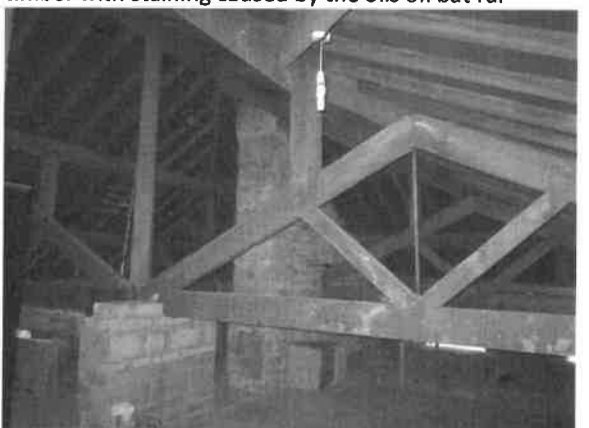
Photo 12: Northern side of roof void showing timber arrangement and large void that will be retained
