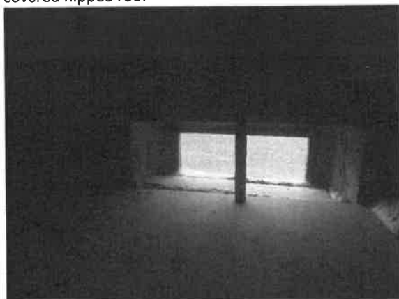
Photo 5: Roof void at Flat 8 showing ceiling crossing the upper section of window
