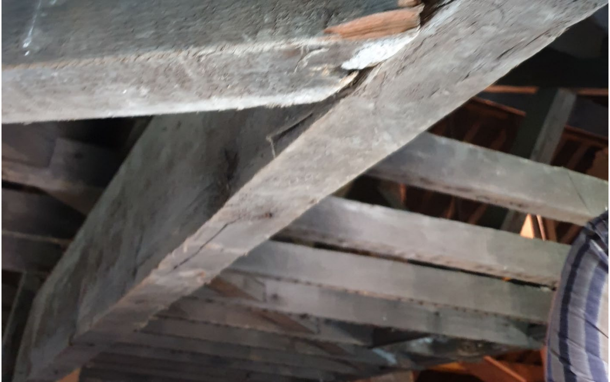
Fig4. Photograph of underside of transvers timbers showing evidence of previously elevated ceiling position
