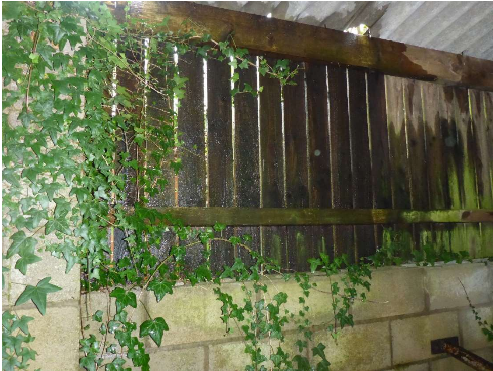
Photo 13: Yorkshire Boarding saturated with water to western side of building.
