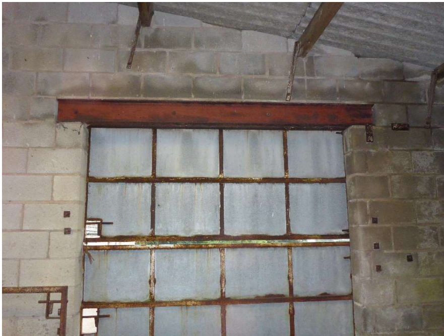
Photo 7: Rusting lintel on internal face of northern elevation
