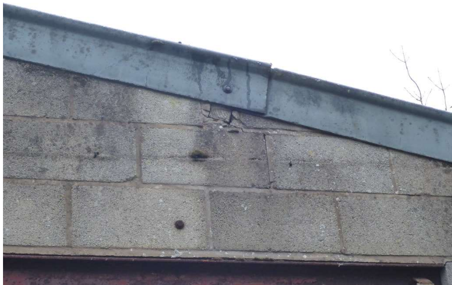
Photo 14: Ends of timber purlins fully exposed on gables of buildings.
