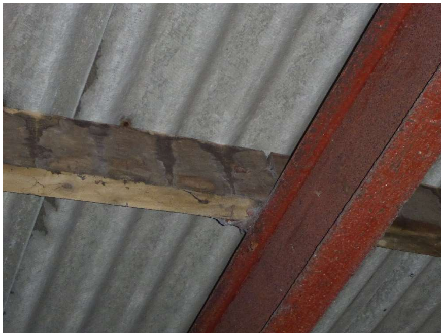
Photo 12: Timber purlins showing signs of water damage.
