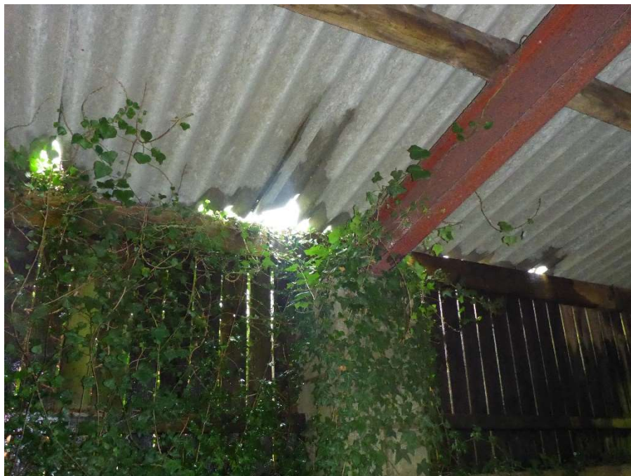
Photo 10: Section of roof sheeting missing and ivy growing within the building.
