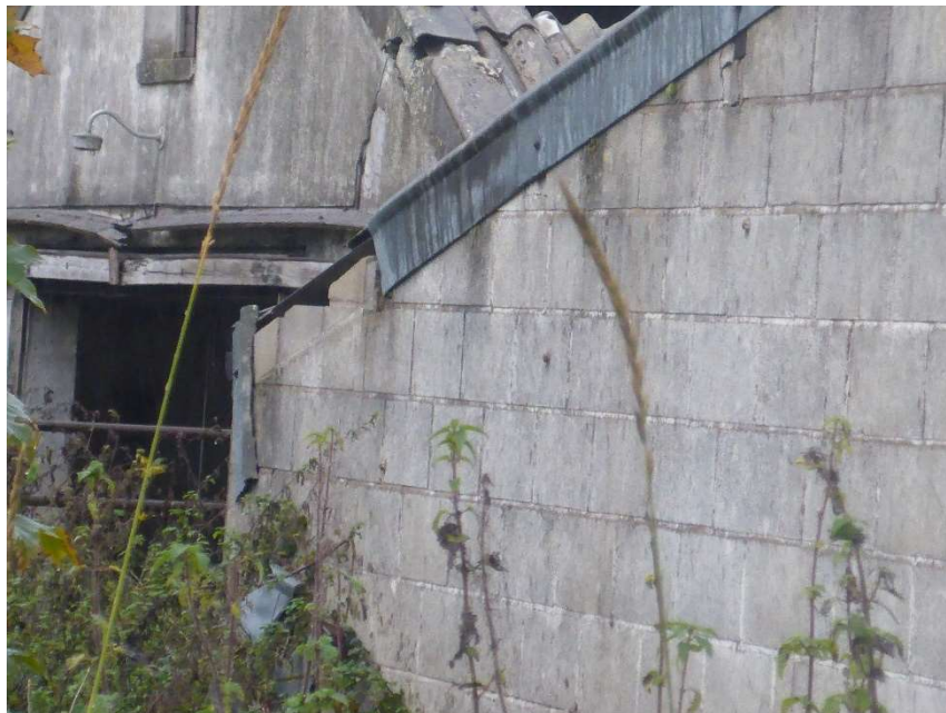
Photo 6: Missing flashing from Southern Elevation.
