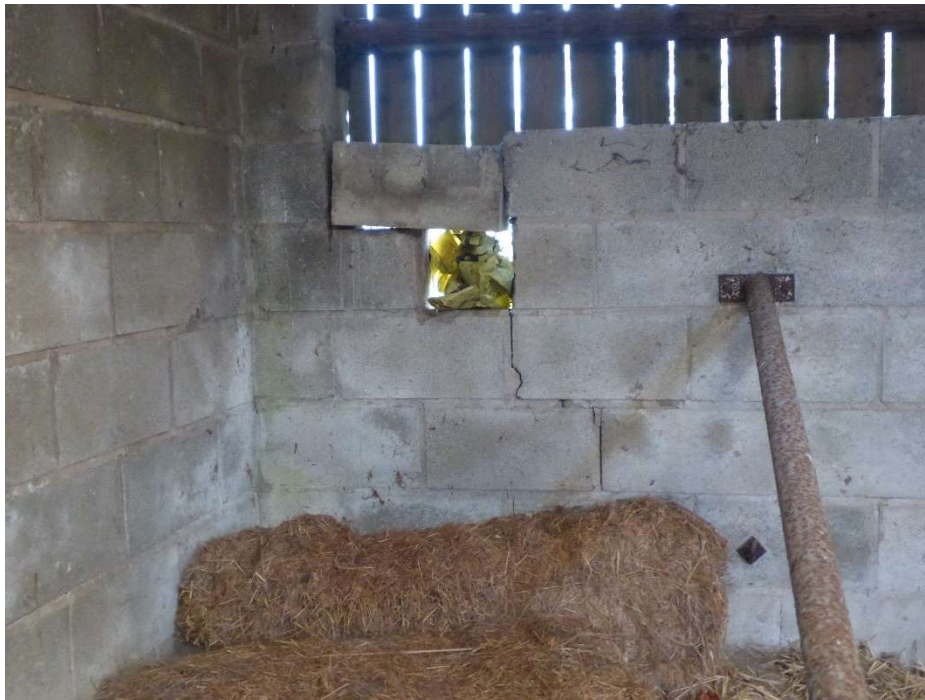
Photo 9: Diagonal cracking/missing blockwork on internal eastern elevation of building
