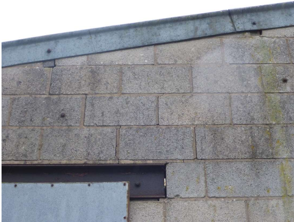
Photo 1: Cracking to North Elevation of the Agricultural Building
