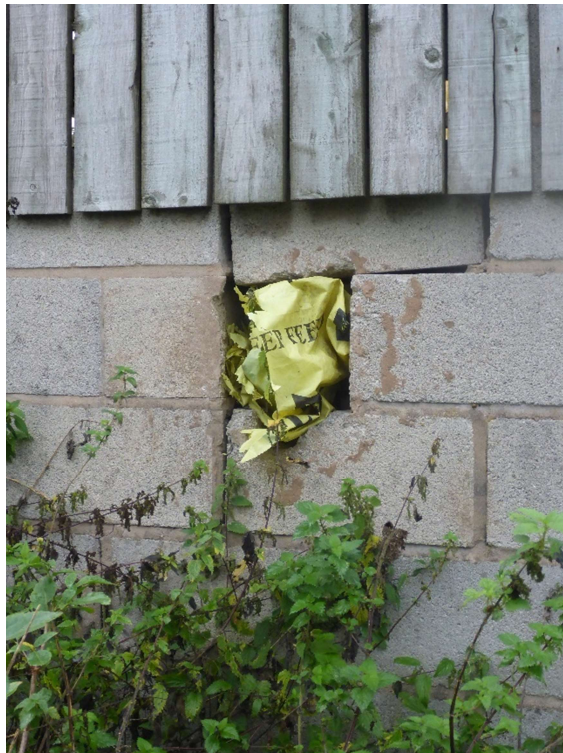
Photo 3: Eastern Elevation of the Agricultural Building showing missing block, localised cracking and loose blocks.
