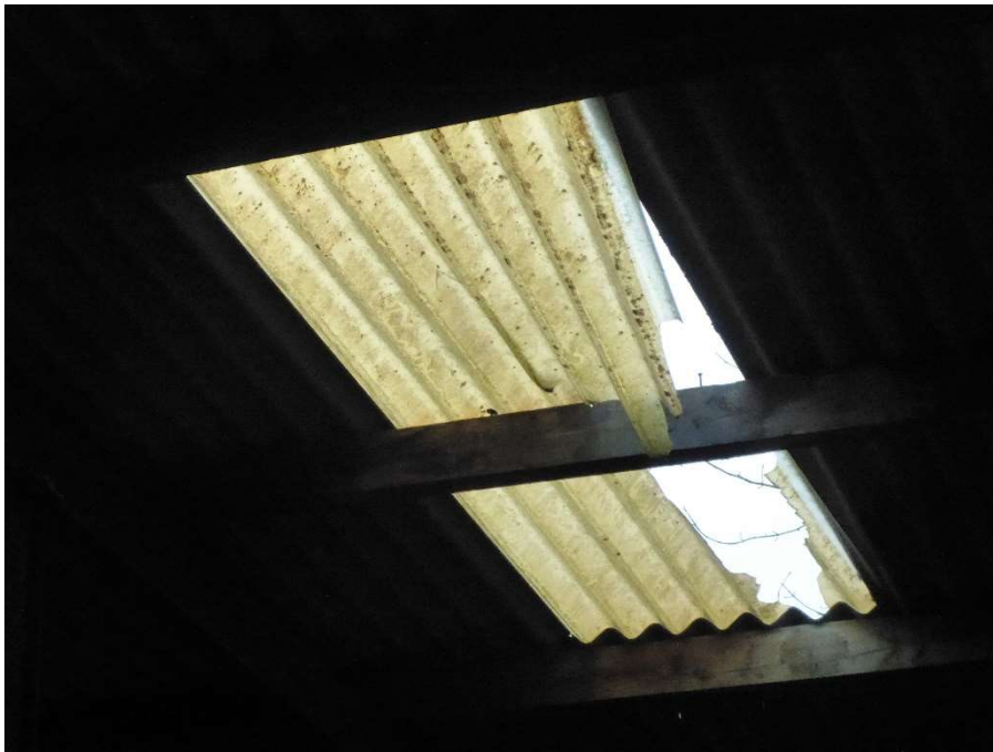
Photo 11: Broken roof light.
