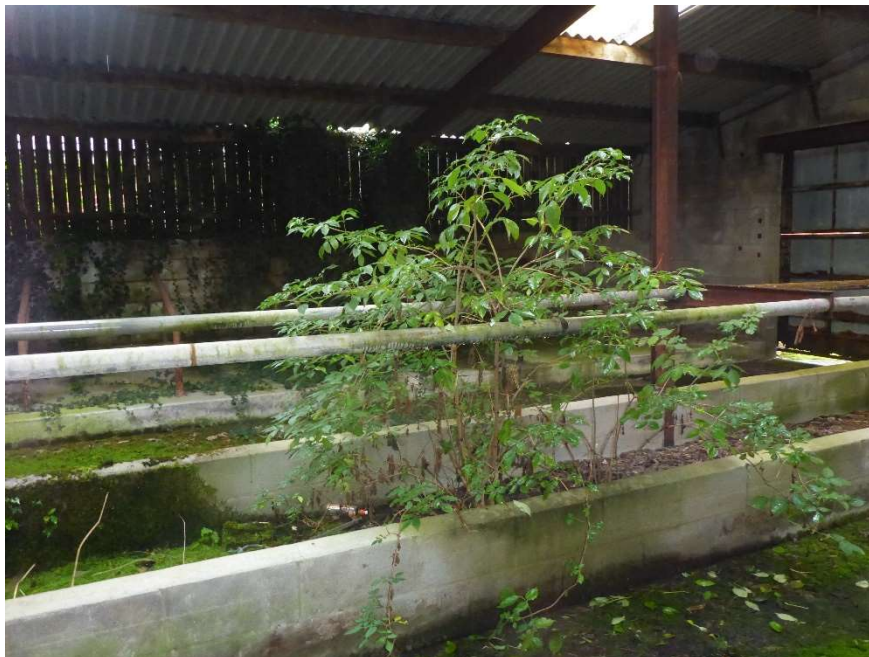
Photo 8: Tree growing in feed passage on western side of building
