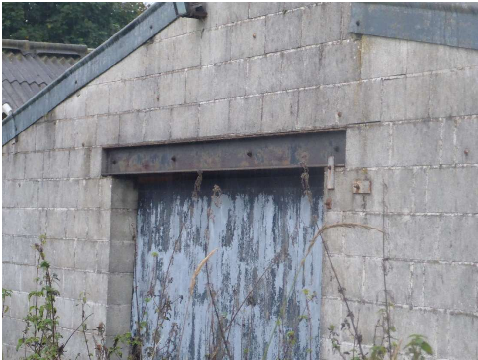
Photo 5: Southern Elevation of the Agricultural Building showing steel lintel rusting.
