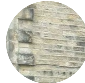
Reference to the projecting quoins at Whins Hall, Sabden (Grade II Listed)
