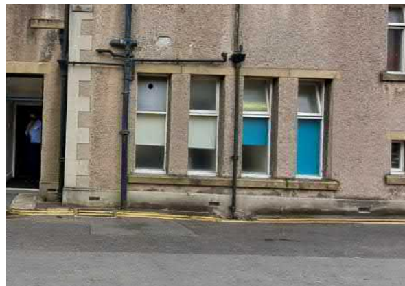
Frosted glass to be replaced with clear to suit new office function
