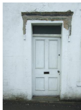
Picture 7 - Original front door with hood missing
