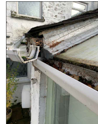
IMAGE 2: FAILED ROOF FLASHINGS/ SEALS
