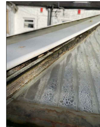
IMAGE 4: FAILED SEALS TO ROOFING SHEETS (DAMP INGRESS)
