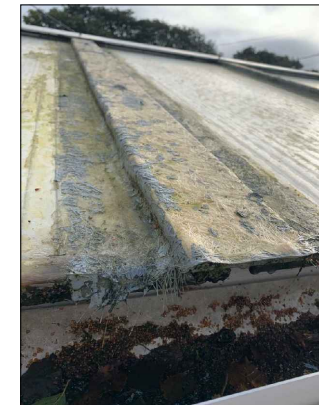
IMAGE 3: FAILED FIBREGLASS ROOF REPAIR
