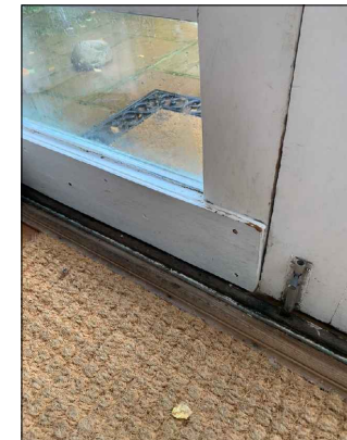
IMAGE 5: DEFECTIVE DOOR THRESHOLD (DAMP INGRESS & AIR LEAKAGE)
