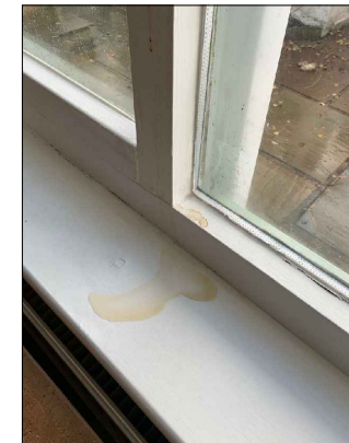
IMAGE 6: INTERNAL DAMP INGRESS AROUND WINDOW & DOOR FRAMES/ SILLS
