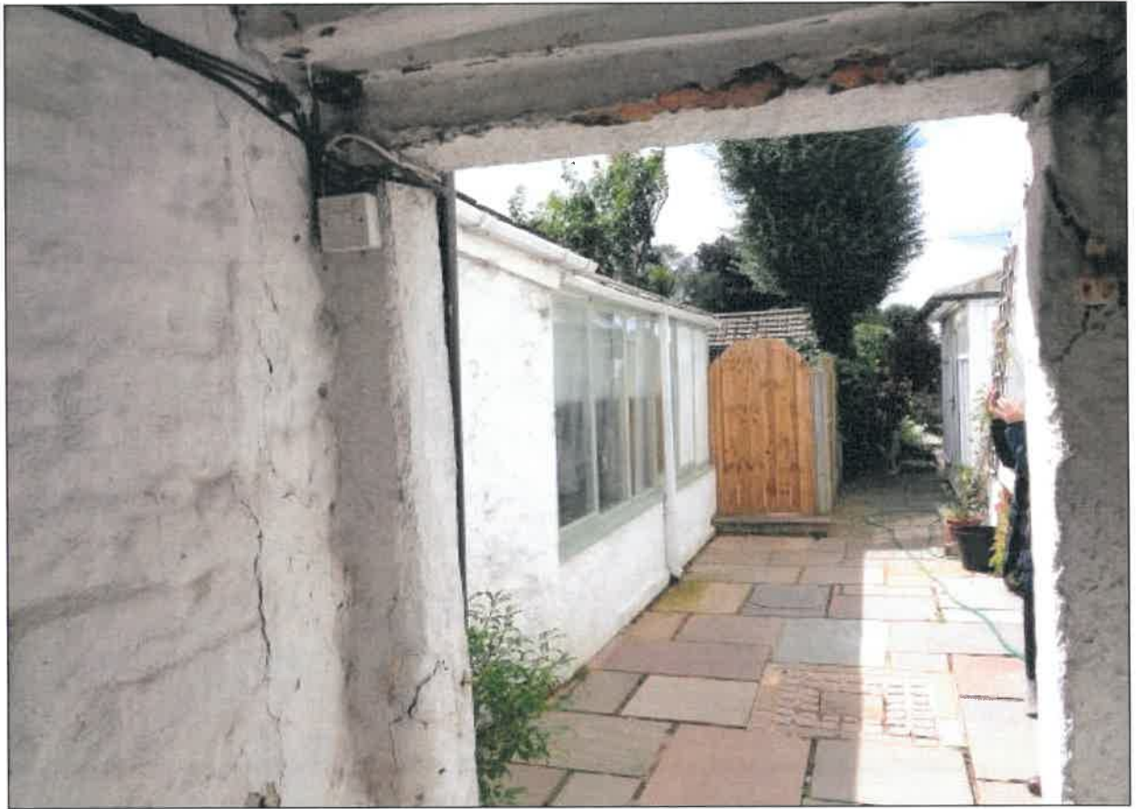
5. Side elevation of the extension seen through the passage from the front
