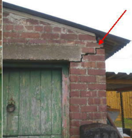
Photo (4)- north east corner of lean -to
