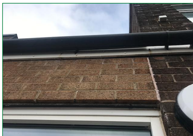
Showing the very narrow gap under the fascia on the two-storey section of the extension.
