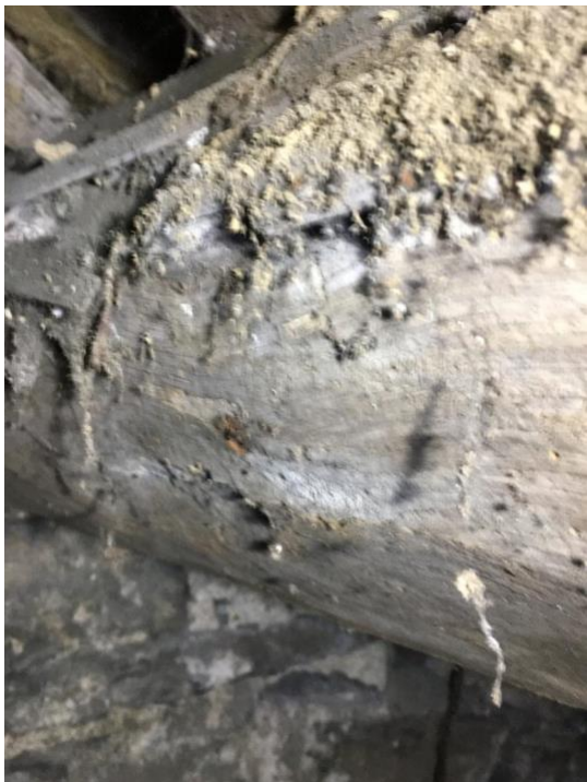
Photo 5: photo showing damaged purlin
