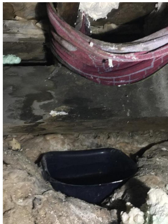
Photo 3: Internal roof space showing water egress
