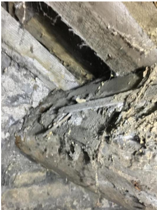
Photo 2: Internal roof space showing worn timber
