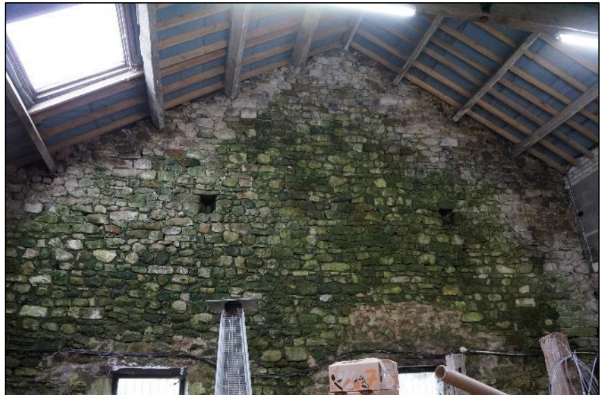
Photo 3: Gable end (west facing) wall of the barn and recently restored roofing materials.
