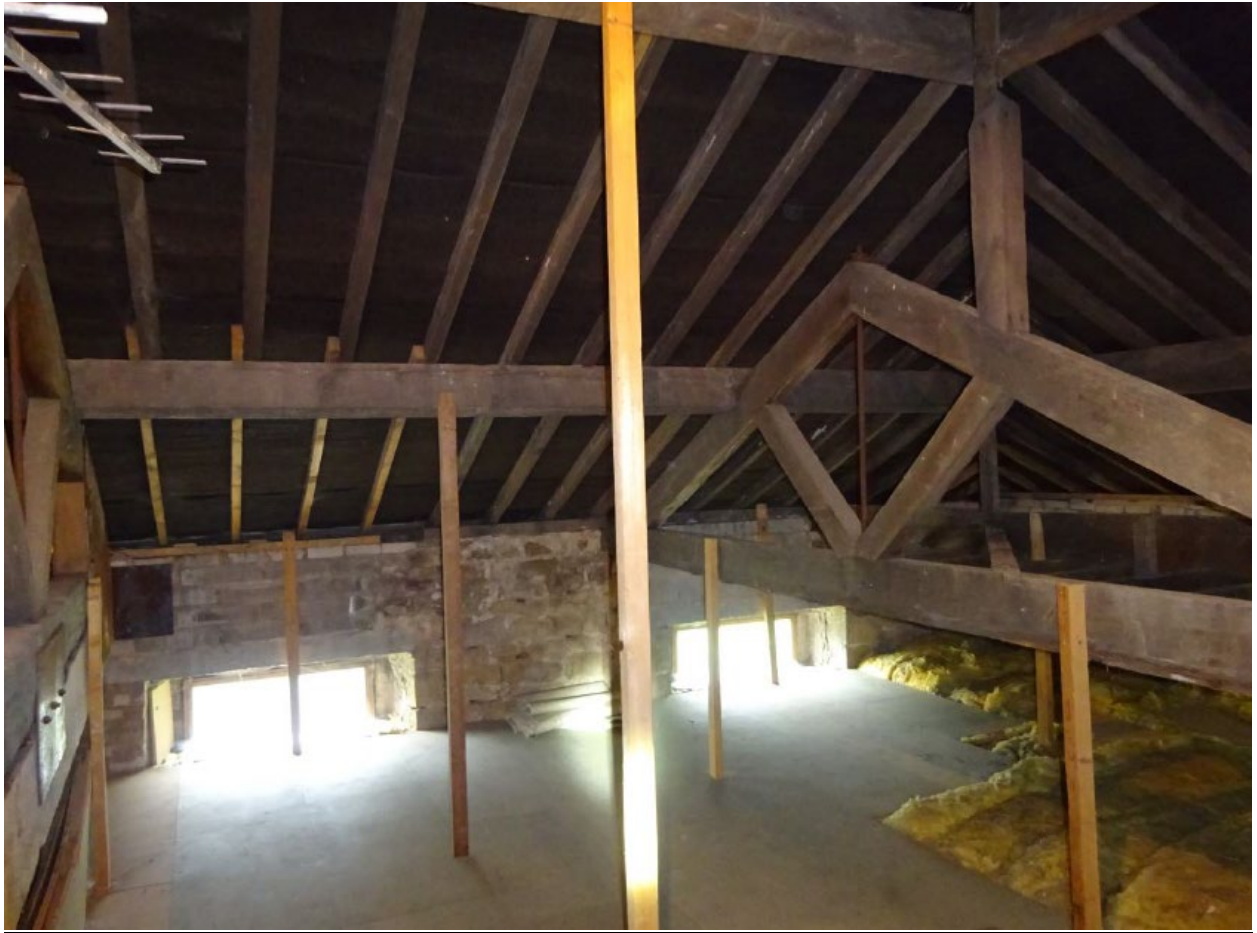
fig 2. Internal view of windows W01 and W02 and shown on elevational drawing.
