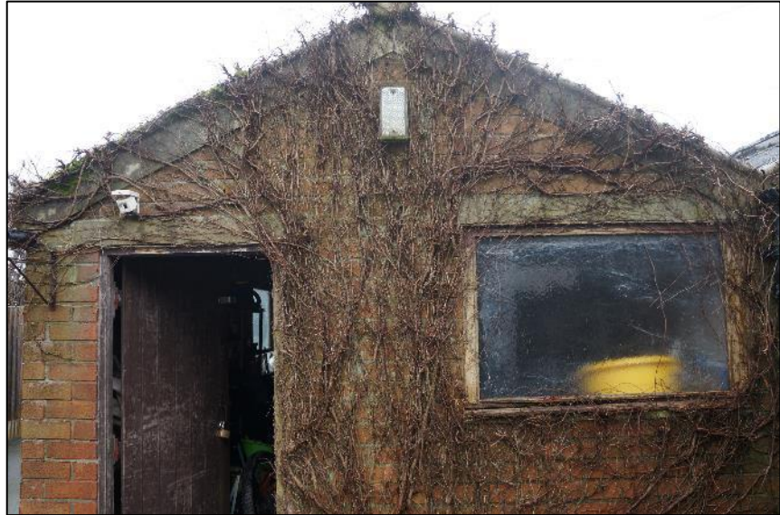
Photo 4: Gable end with creeper growing over the fascia.
