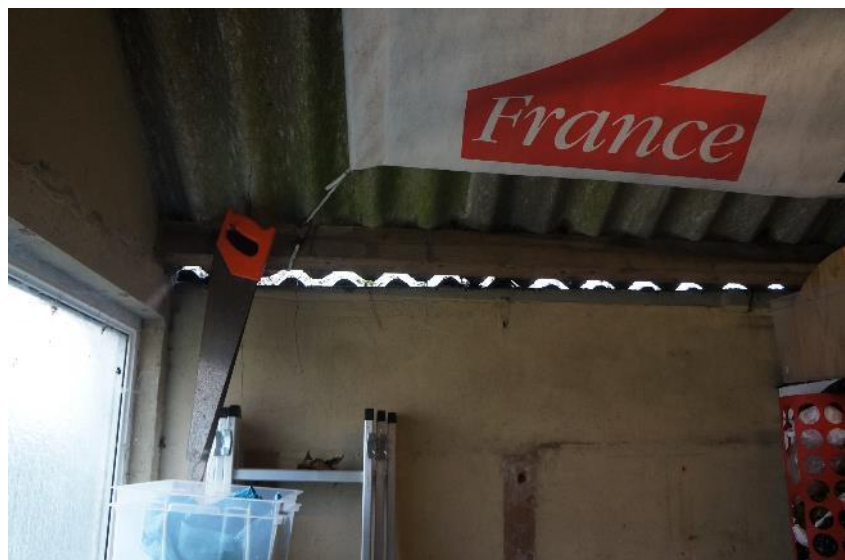
Photo 5: Gaps to the exterior where the roof materials no longer meet the walls.
